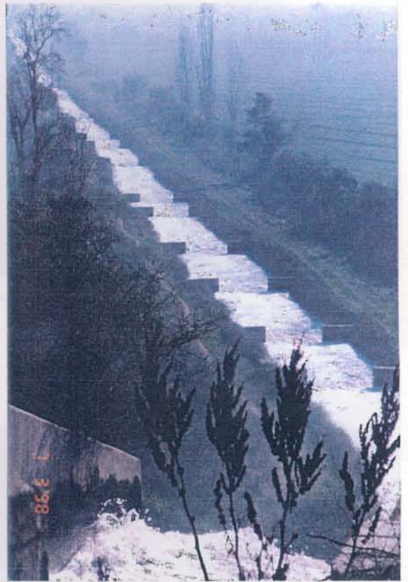
▲ Energy dissipator in the midstream of Mercedes canal
