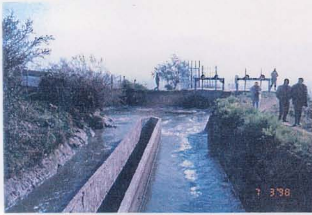
▲ Intake facilities in the midstream of the Mapocho River (Mallarauco canal)
